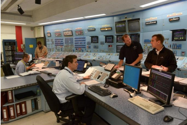
Exhibit 2.12 - PLGS control room
